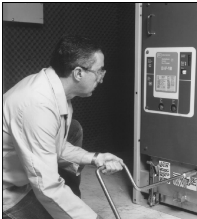
Figure 4-13 Levering 5 kV Breaker to Connected Position
