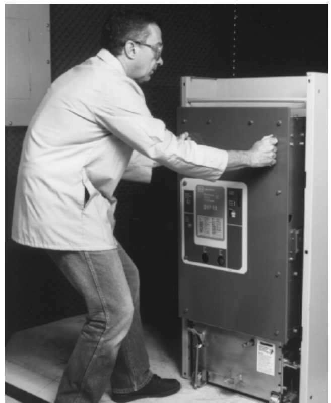
Figure 4-9 Positioning of 5 kV DHP-VR Breaker
