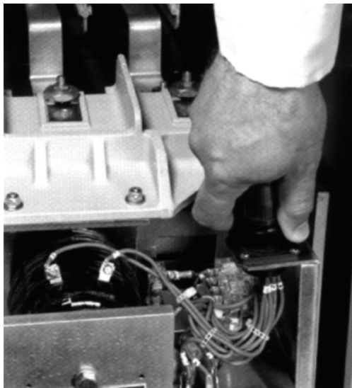
Figure 11 Disconnecting Contactor Control Cable
