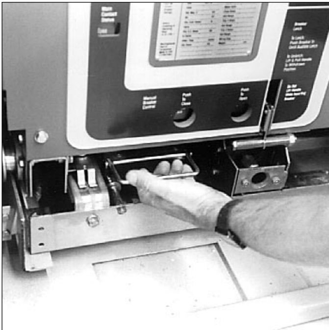
Figure 4-5 Pulling Secondary Disconnect Cage to Engage Secondaries in TEST Position
