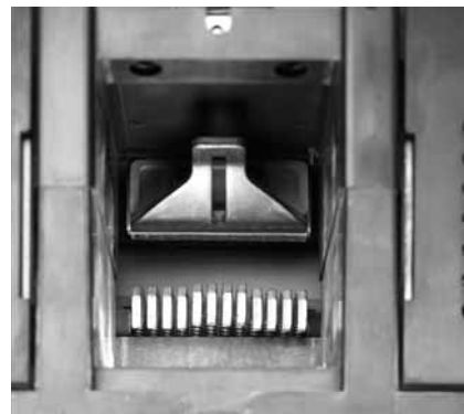
Magnum DS breaker contacts (arc chutes removed)
